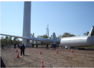
One of the final wind towers under construction at the 99 MW Greenwich windfarm near Dorion. Environment North members Scott Harris, Lucy Laframboise, Charlene Rogers and Kerstin Muth visited the nearly completed windfarm in October 2011.
