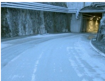
Entrance to Finland’s nuclear waste disposal site, under construction From the film “Into Eternity”
